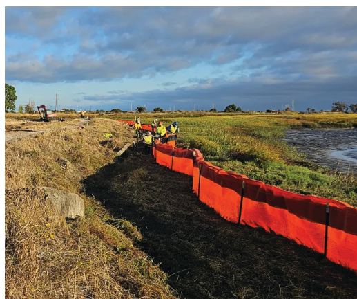
▲ Workers protect Harbor Marsh by installing temporary fencing at the edge of the Horizontal Levee restoration. Credit: City of Palo Alto
