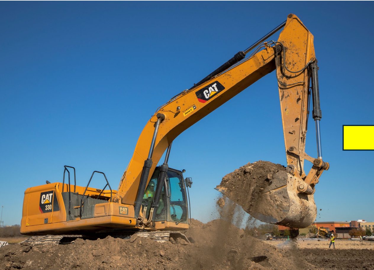
Excess upland construction soil
