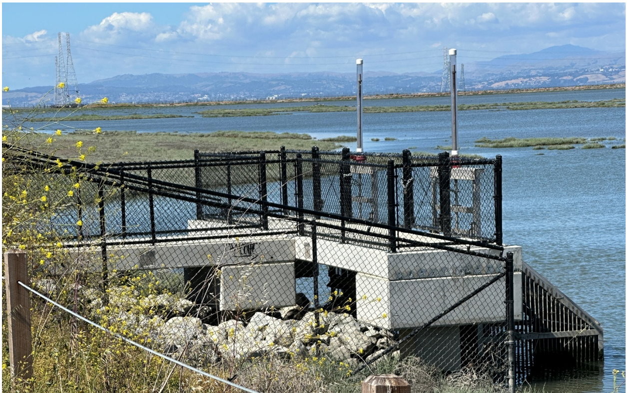
Figure 4-13: A Water Control Structure That Interconnects Ponds
