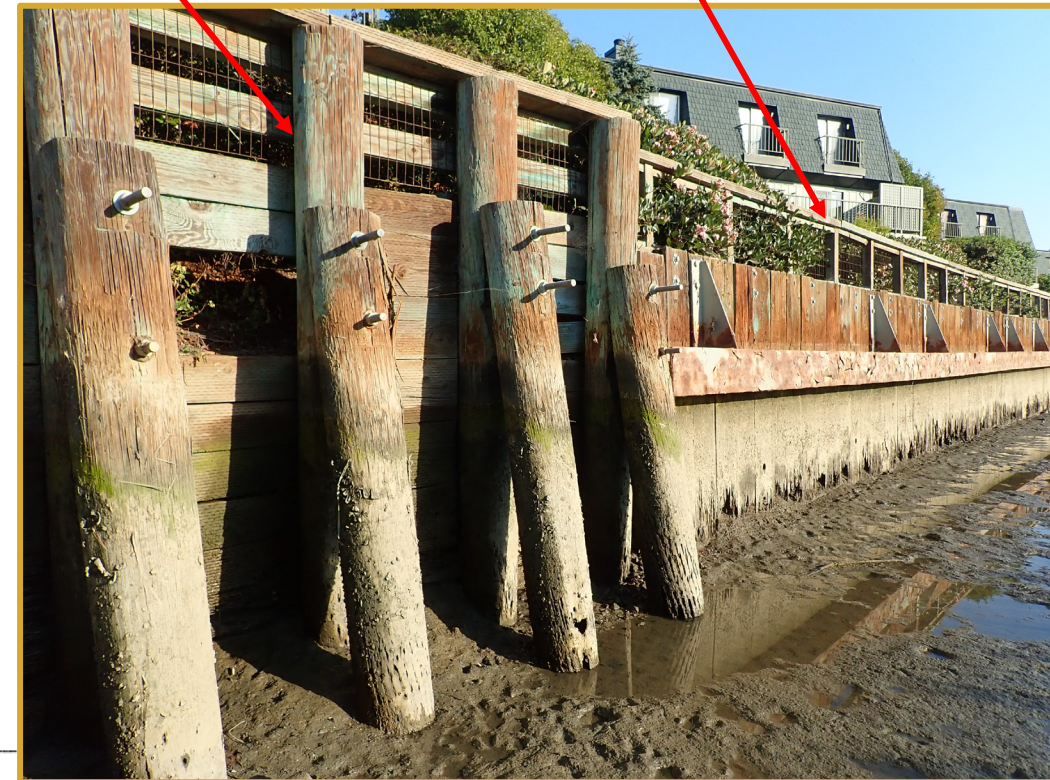
1989 Seawall Repair (Existing Condition)
